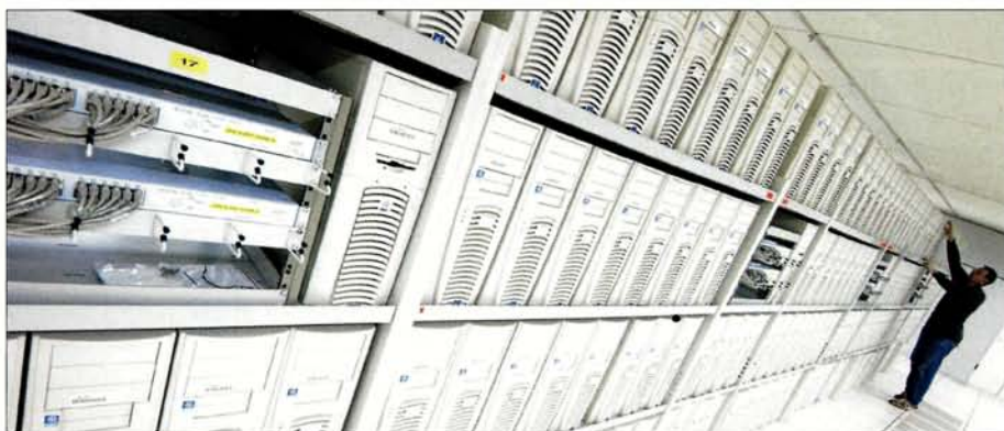
A view of the new machine room in the basement of CERN's computer centre.
